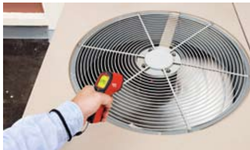
Measure efficiency of heat dissipation to reveal and locate thermal losses in the flow system.
